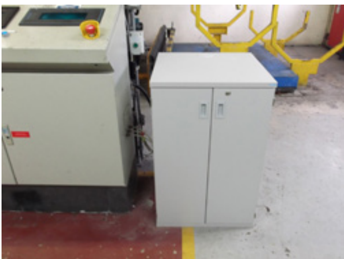
Figure 4: EDAS Cabinet provided by the Operator
