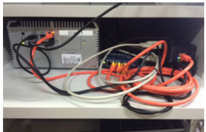
Figure 6: EDAS System installed in operator cabinet, showing the Euratom computer (left), network switch (middle), and two EDAS branching units (right)
